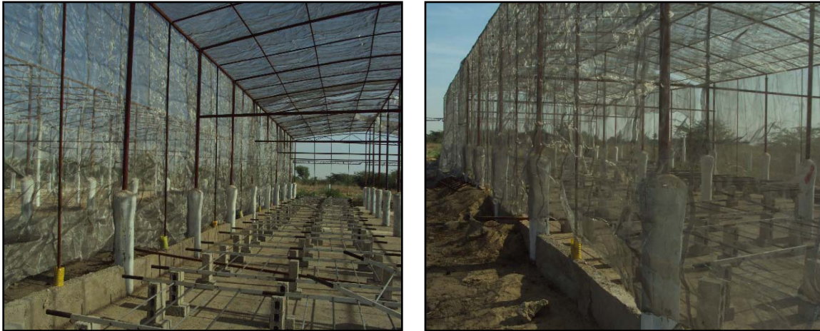
Pictures of a Screen House being erected in Karachi with the support of ASF for production of fruit plant nursery under insect-free environment.
