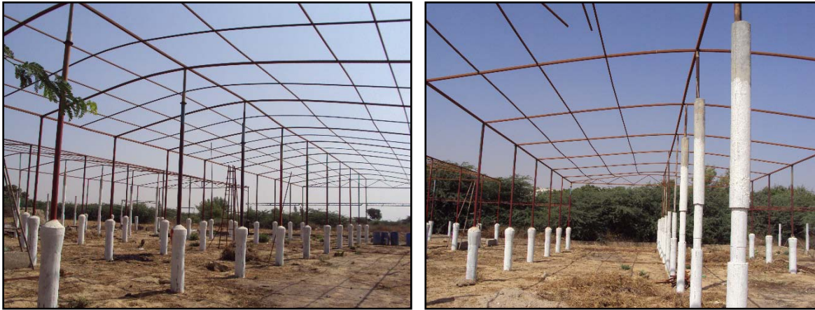
Pictures of a Screen House being erected in Karachi with the support of ASF for production of fruit plant nursery under insect-free environment.
